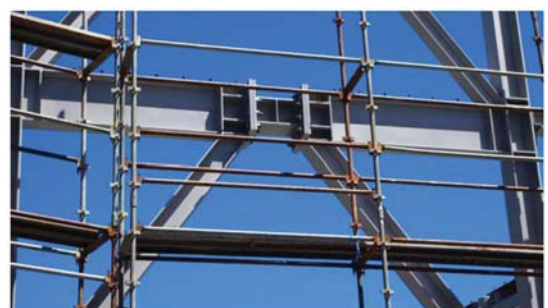
Fig. 6. Close-up of replaceable link in an eccentrically braced frame. (Image by Michel Bruneau.)
