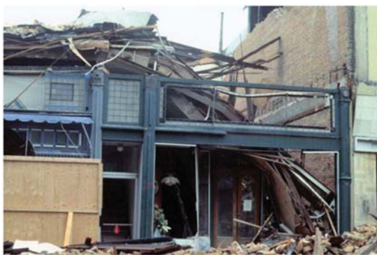
Fig. 7. Damage to low-rise building in Santa Cruz, California, due to collapsed parapet from adjacent building during 1989 Loma Prieta earthquake. (Image by Michel Bruneau.)
